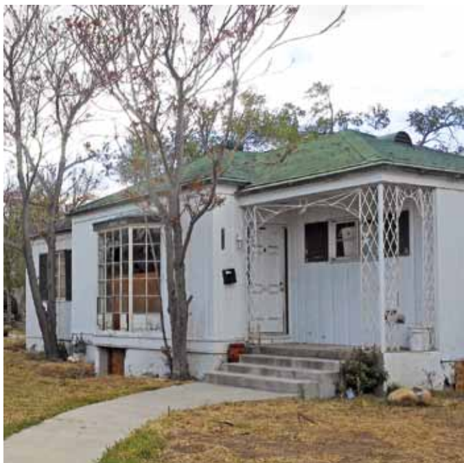
The deteriorating El Reno apartment home at 1461 Lander Street in 2016 with chipped paint, broken and boarded up windows and dried up lawn and plants. The home is pictured on page one in 2004 in a much better state. Photo by the author.
